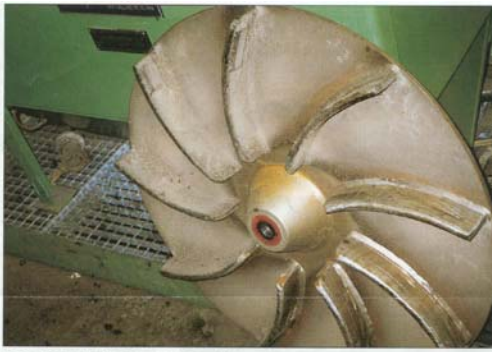
Fig. 5: Fan impeller showing wear after 1 week of operating time
