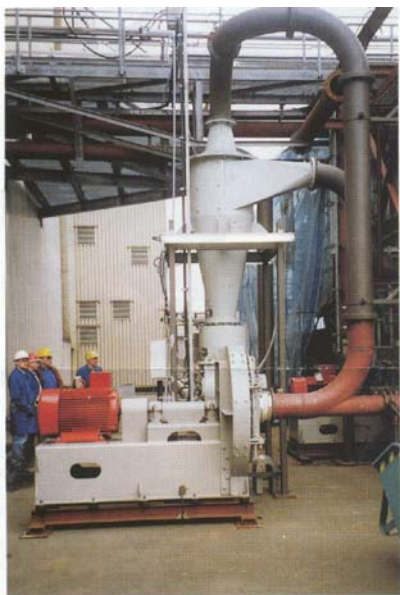
Fig. 3: Cyclone, fan and piping
